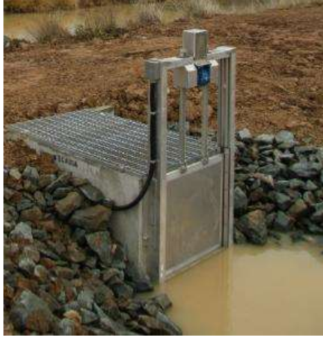
Photo 23 Automatic slide gate installed on box culvert opening
