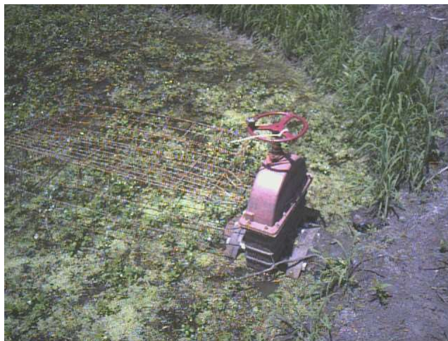
Photo 10 Slide gate valve
