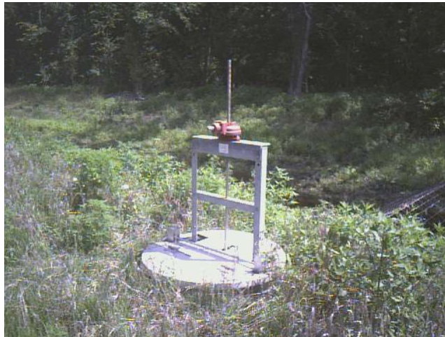
Photo 3 Stop log-slide gate combination water control structure
