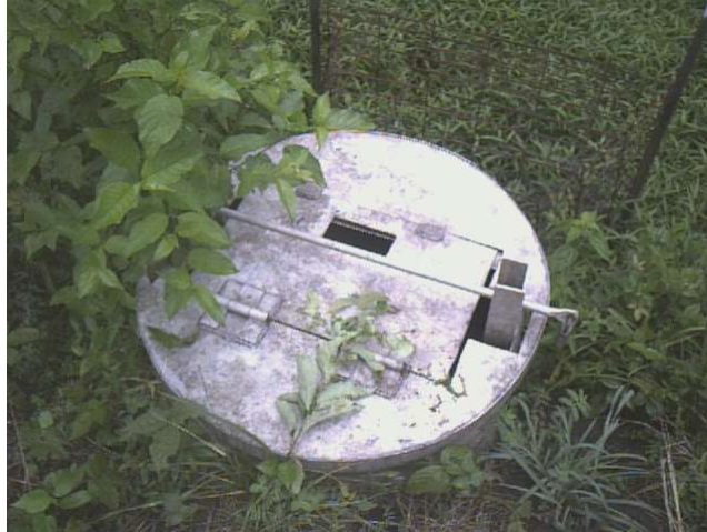
Photo 2 Stop log riser with metal cap
