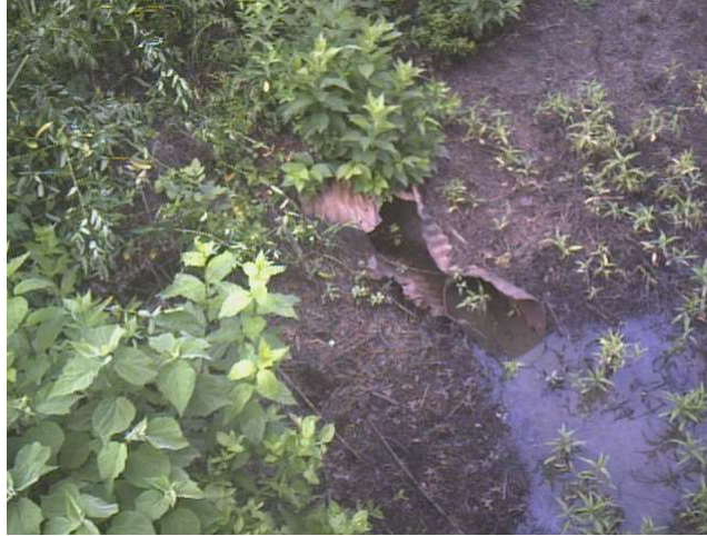
Photo 7 Damaged corrugated metal pipe
