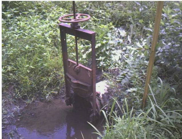
Photo 9 Slide gate mounted directly on pipe
